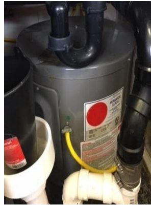
Tank water heater
