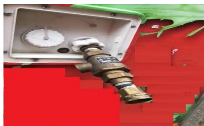
Backflow preventer installed on exterior of unit for connection of public water line
