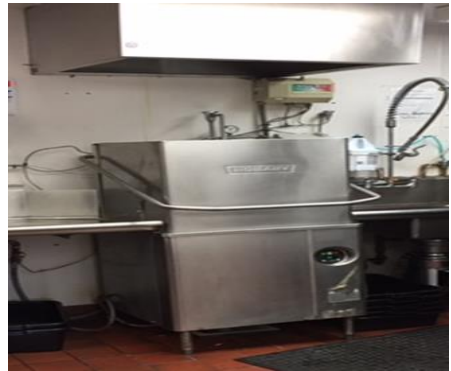
Type II hood over heat/moisture producing dishmachine
