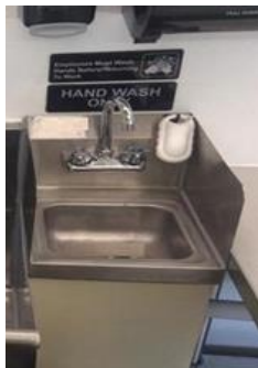
Fixed standalone handwash station
